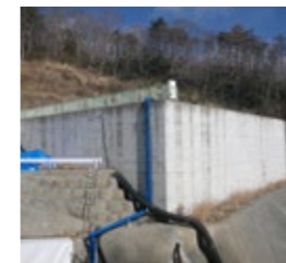
Leachate regulation tank
