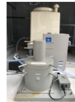
Continuous measurement system for groundwater radioactivity concentration
