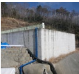
Leachate regulation tank
